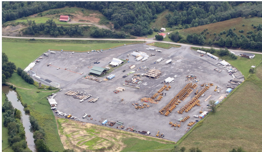
ACP contractor yard between WV 92 and Knapps Creek south of Frost in Pocahontas County. This yard was developed in the summer of 2018.
