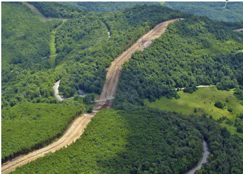
Point Mountain in Randolph County obtained on July 28th. The ACP corridor has been cleared and the trench has been excavated. This work occurred after the Fourth Circuit Court of Appeals voided the Incidental Take Statement for the ACP.
