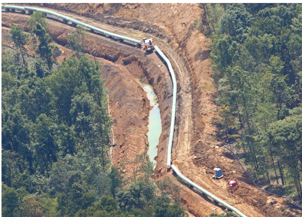
Laurel Run in Upshur County, 2018. Pipe strung and welded adjacent the excavated trench in the Buckhannon River area of Upshur County. Dominion moved over 30,000 feet of pipe to the ACP construction corridor after the required Incidental Take Permit was voided by the Fourth Circuit Court of Appeals in May 2018.
