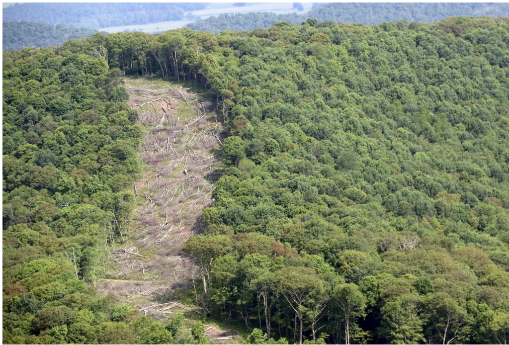
Trees were felled for the ACP in early 2018 in this section of the National Forest on Allegheny Mountain along the Virginia-West Virginia border. The Forest Service initially raised concerns about the hazards of pipeline construction on the extreme slopes in this area. These concerns were seemingly forgotten by the time the Forest Service granted a Special Use Permit for the project.
