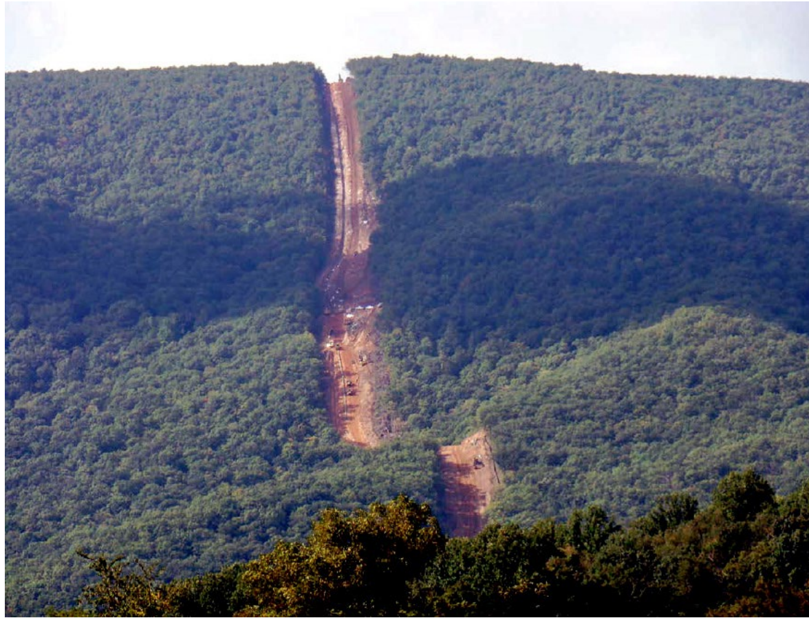
Example of a pipeline right-of-way corridor through the mountains. (Photo courtesy of Rick Webb)
