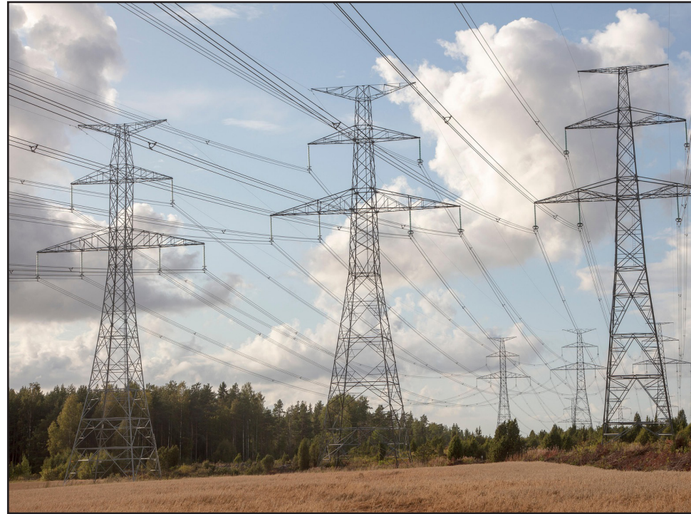
Transmission lines similar to those of the proposed MARL and Valley Link projects.
